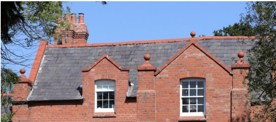
Examples of local roof material. Note the detail brick and timber work of the gables.
